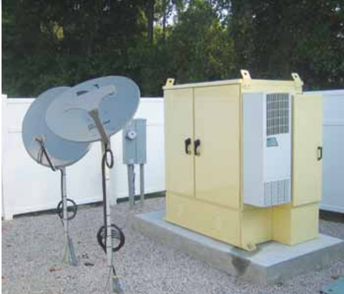
Figure 2: Connexion Head-End Cabinet
